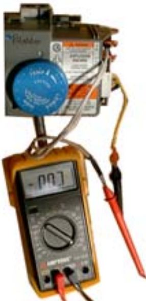
Measuring flame signal
