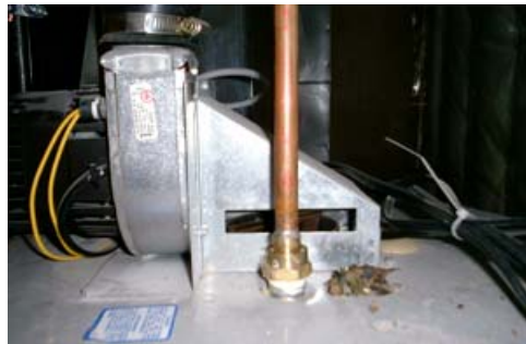
Ensuring draft hood air inlets are free of debris and obstructions
