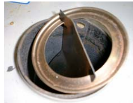
Baffle out of correct positioning
