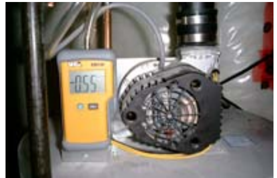
Measuring draft at blower with electronic manometer
