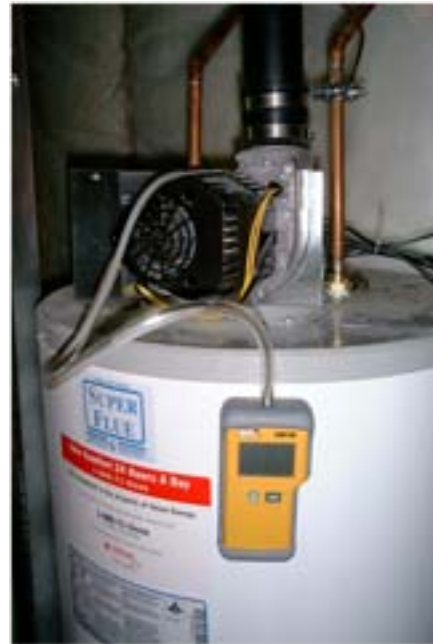
Measuring draft at blower with electronic manometer
