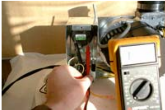
Checking air switch operation with Ohmmeter
