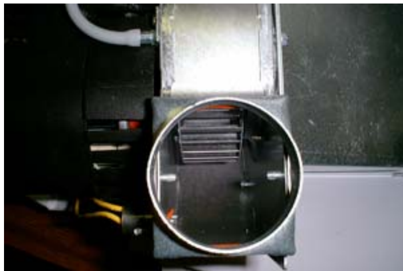
Ensuring blower is free of dirt and dust build up
