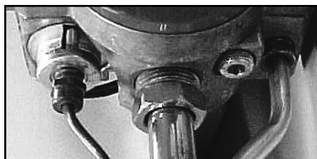
Figure 12 - Gas Pressure Check
